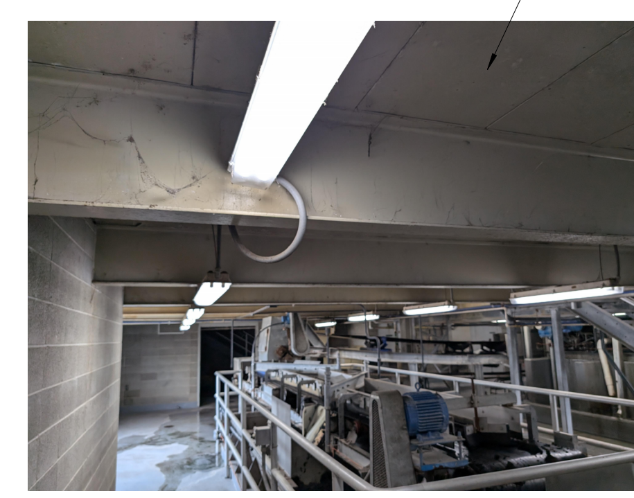
SECOND FLOOR CONVEYOR
